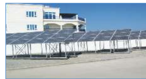
Middle East Desalination Research Center – MEDRC (Oman) - 15Kwp Solar Powered Grid Connect System
