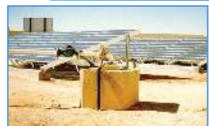
Field (Oman) Solar Water Pumping System
