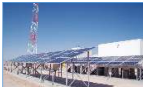
PDO (Oman) 2.5Kwp SPS for Instrumentation & Control System
