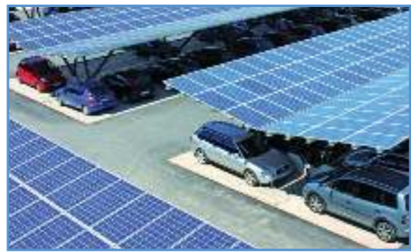
Port Authority, DUQM (Oman) SPS Car Parking – 60Kwp
