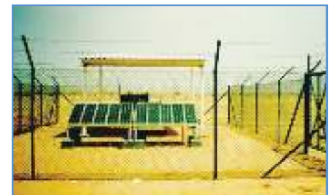
PDO (Oman) 6Kwp SPS, CATHODIC, PROTECTION x 12 sites
