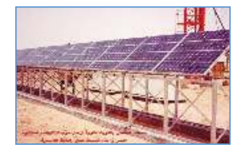
Telecom (Kuwait) 2.54Kwp SPS Microwave Repeater Station
