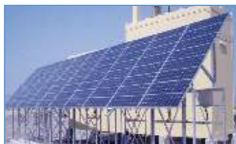
PDO(Oman), SPS - BLOCK VALVE STATION
