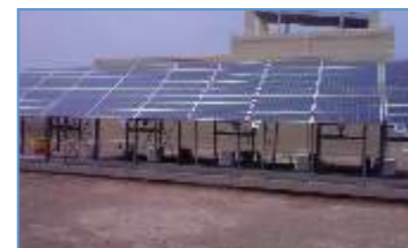
OGC (Oman), 123.5Kwp (Duqm) & 182.24 Kwp (Liwa) SPS for Launcher & BVS
