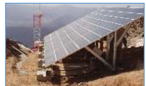
PDO (Oman), 25Kwp SPS Telecom Station
