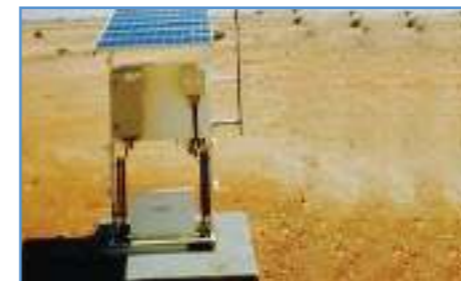
PDO (Oman) 27Kwp SPS MSV MOTOR & WELL HEAD RTU x 44 Sites
