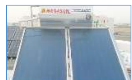
GU Tech – Eco House (Oman) Solar Water Heating System
